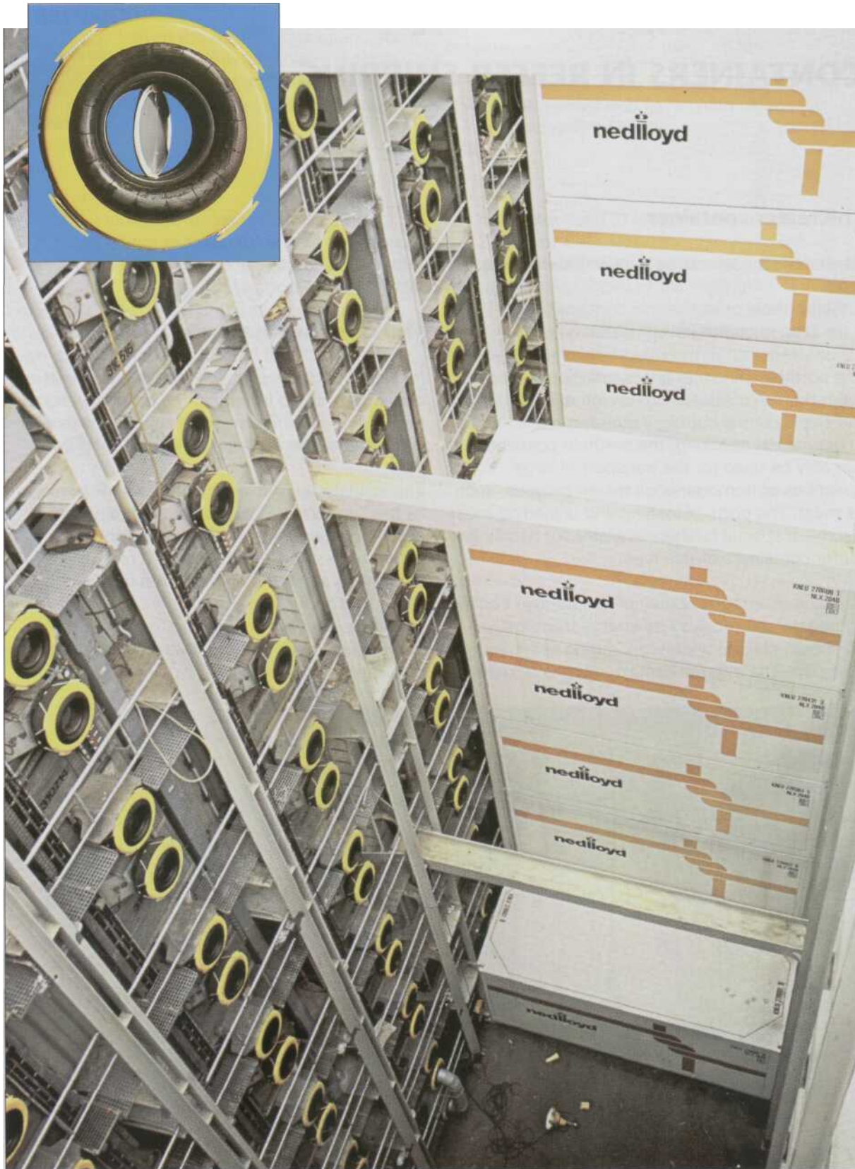
"The vertical Ducts system"
