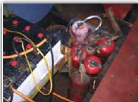
Figure 93: Fire Extinguishers on Low-Standard Tanker Barge
