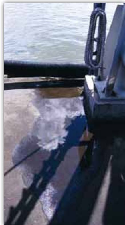
Figure 62: Minor Spill Probably Due to Gasket/Flange Leak
