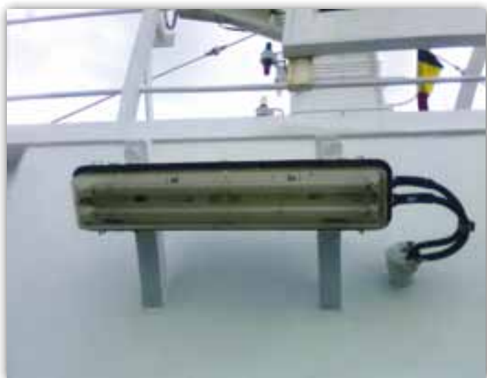
Figure 85: Standardized Explosion-Proof Deck Light
