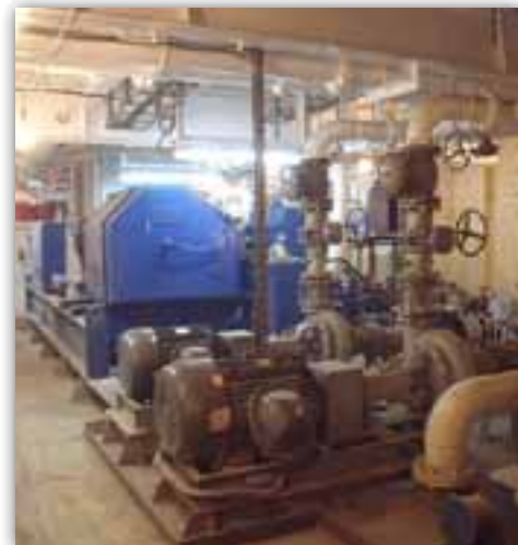
Figure 76: Cargo Pump Room
