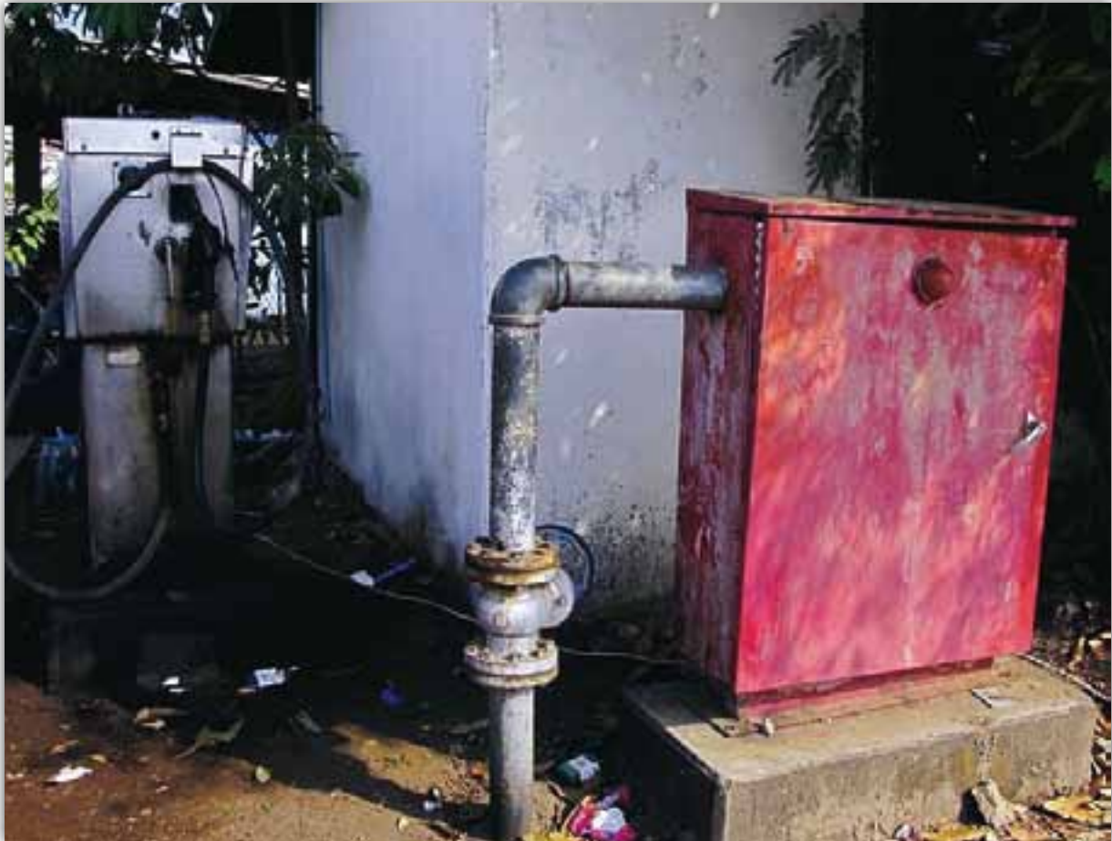
Figure 67: Poor Maintenance of Port Equipment
