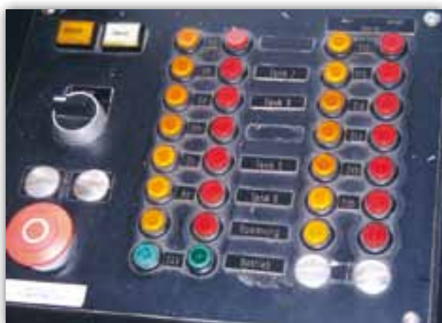
Figure 80: Tank-Capacity Alarm Panel
