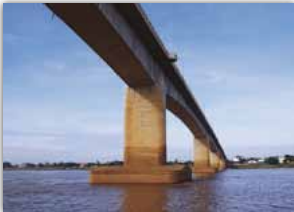
The bridge at Kampong Cham does not have air-clearance indication for shipping
