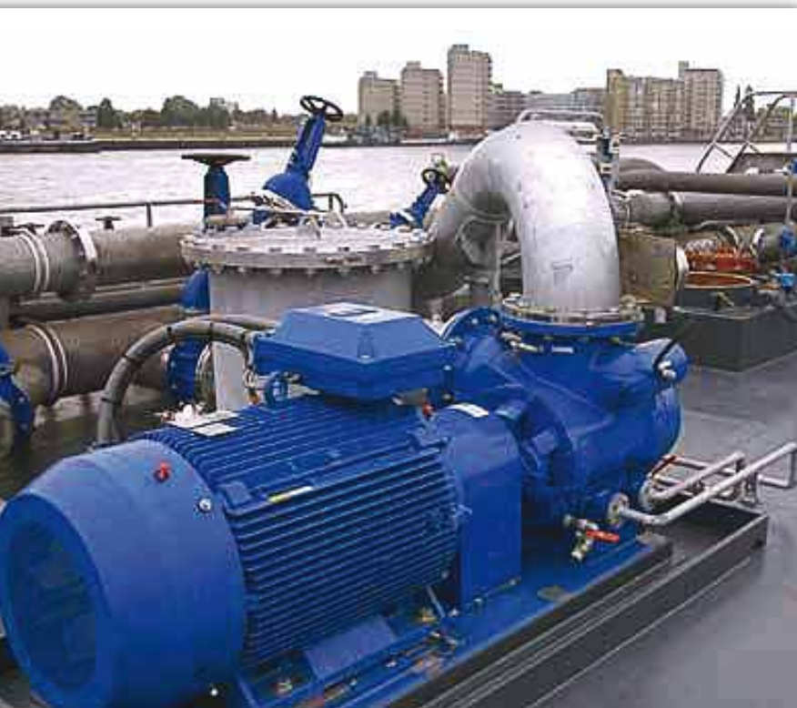
Figure 75: Cargo Pumps on Deck
