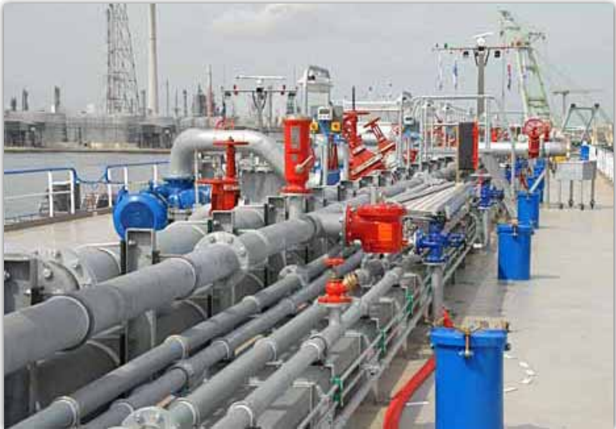
Figure 77: High-Standard Cargo Pipes
