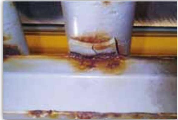
Figure 18: Corrosion at a Contact Point at a Pipe Support 7
