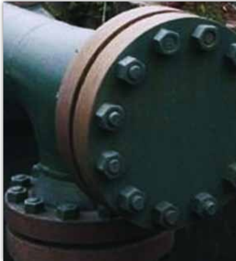
Figure 16: Correctly Blinded Cargo Line
